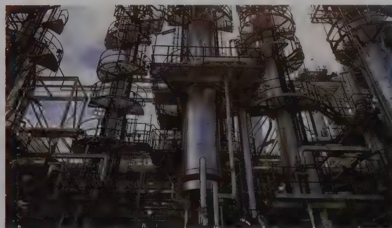
● Figure 8.6 The skyline of an oil refinery is dominated by fractional distillation columns.
